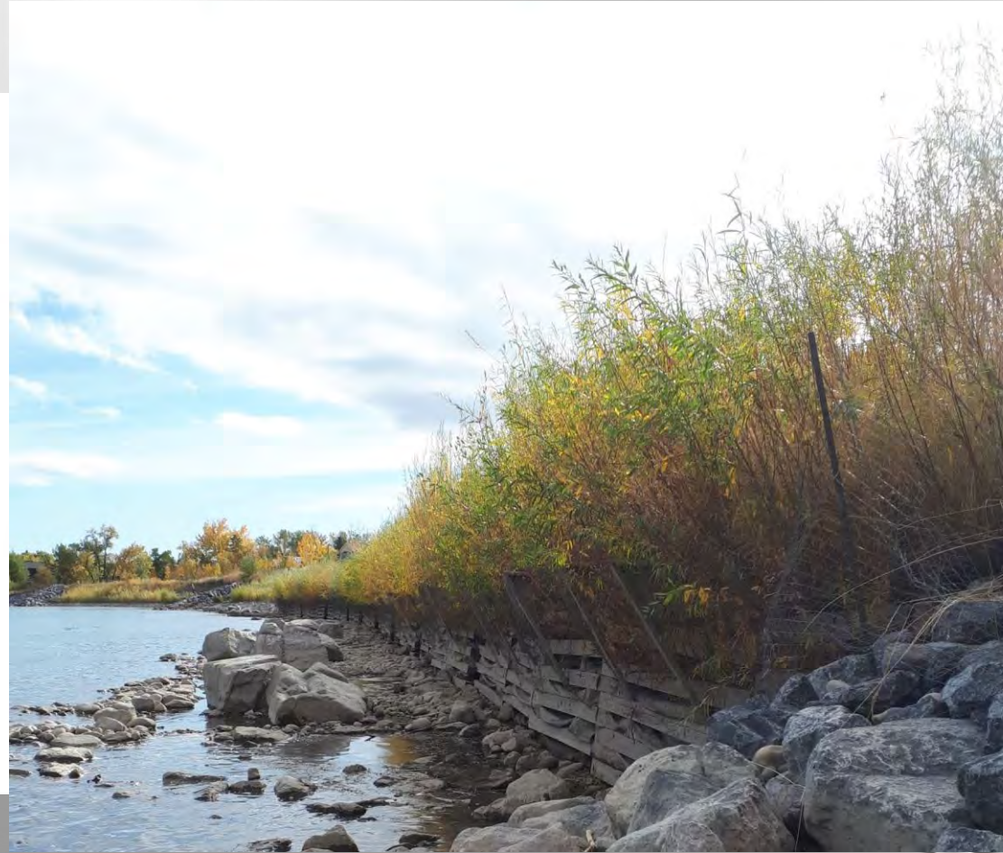
Living Crib Wall for Bank Protection (City of Calgary Bioengineering Demonstration and Education Project)
