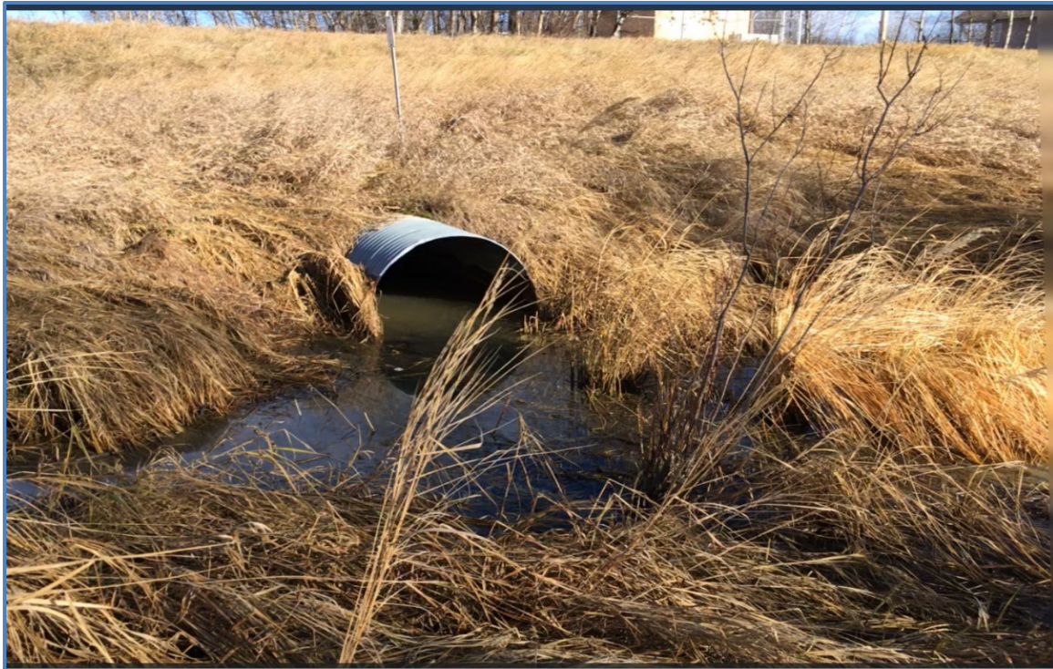
Figure 4.5b - October 24, 2017, Photo Showing Vegetation and Standing Water Restricting Outflow at Downstream End of Antler Lake Outlet Culvert.
