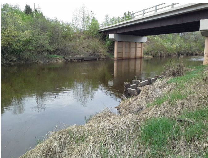
Photo No.: Photos-20180516-202538.jpg Description: Erosion control?
