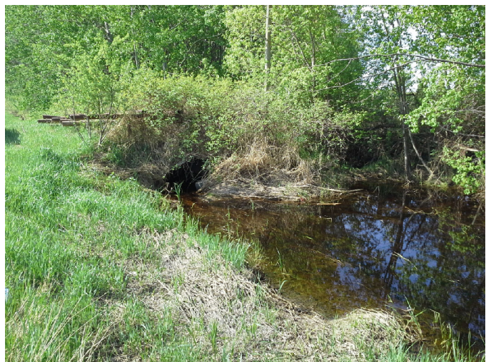
Photo No.: Photos-20180518-165939.jpg Description: Culvert downstream from farm access road 20m downstream
