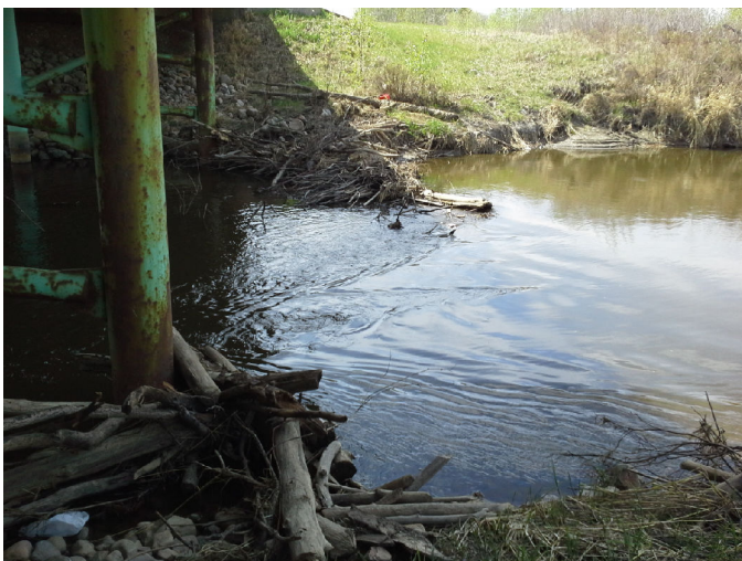
Photo No.: Photos-20180514-214037.jpg Description: Debris build up
